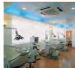
4-way Ceiling Cassette Type
